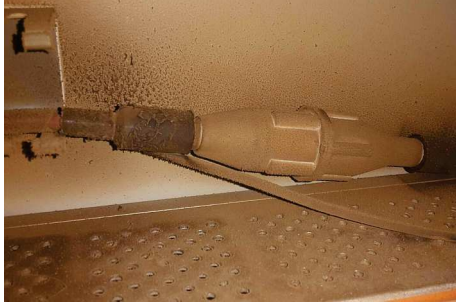
The high-voltage connector between the power supply and the tube MUST be kept dust-free & clean at all times.
