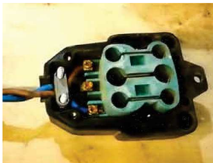
This is an Unsafe connection diagram for an extension lead, where the Live and Neutral wires are swapped at each socket.
